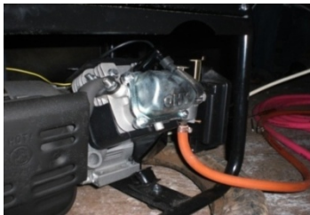
Gambar 10. Generator berbahan bakar gas metana
