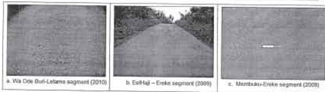
Figure 9. Major Damage on The evaluated Road Segments
