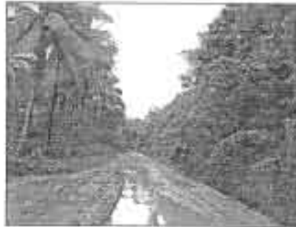
Figure 1. Road Condition of Unpaved Road on North-South Corridor of Buton Island
