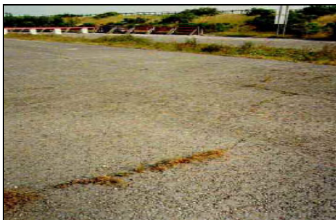
Figure 3 The reflection crack on the road that has never been passed by vehicles traffic for 12 years
