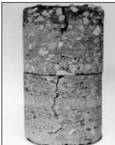
Figure 1 Reflection crack propagation on road pavement
