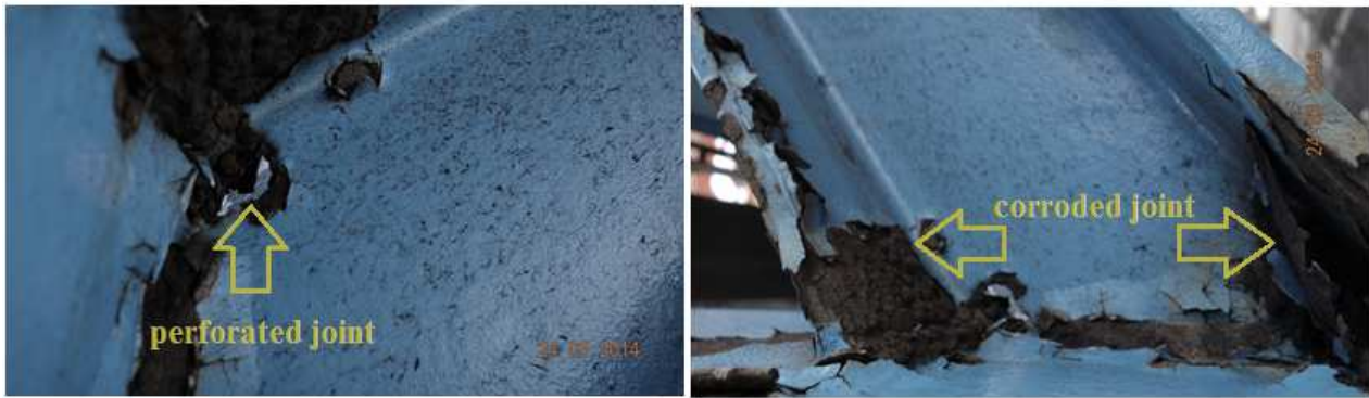
Fig.2 Corrosion attacks on joint areas.
