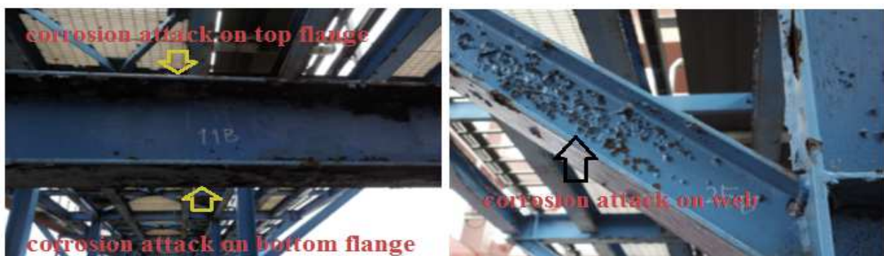
Fig.1 Corrosion attacks on top and bottom flange (left) and on web (right).
