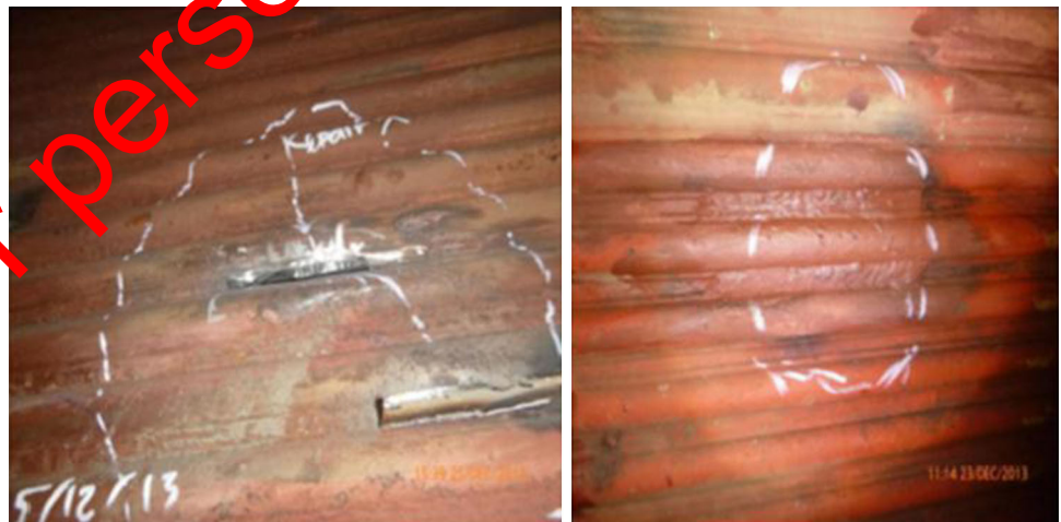
Fig. 1 The leaking water wall tubes in a 660 MW supercritical boiler
